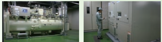
Facilities at Fujinomiya Factory (Left: high-efficiency turbo refrigeration unit; right: inverter chiller refrigeration unit)
